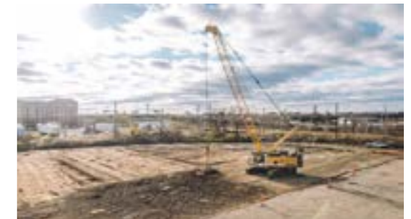
Flat Rock Data Center (France)
