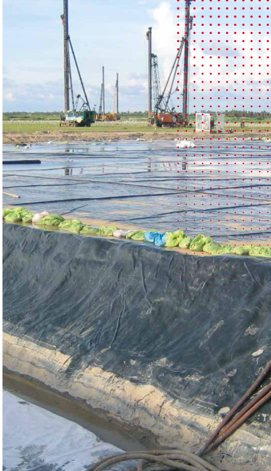
▲ Vietnam - Ca Mau Power Plant
