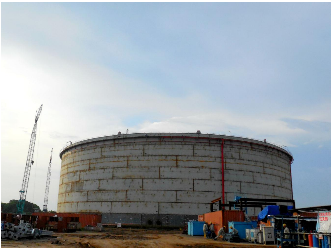
Figure 1: View of Additional Naphtha Storage Tank FB 1801E– Latest Photograph
